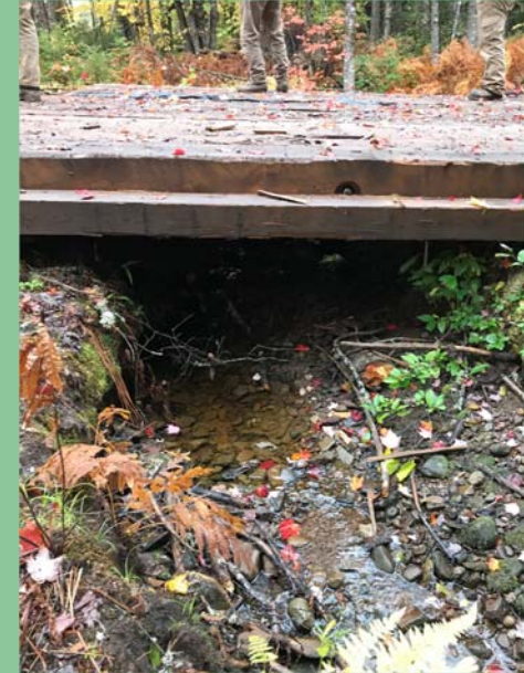
A temporary crossing used during harvest operations showing protection of stream banks and water quality.
