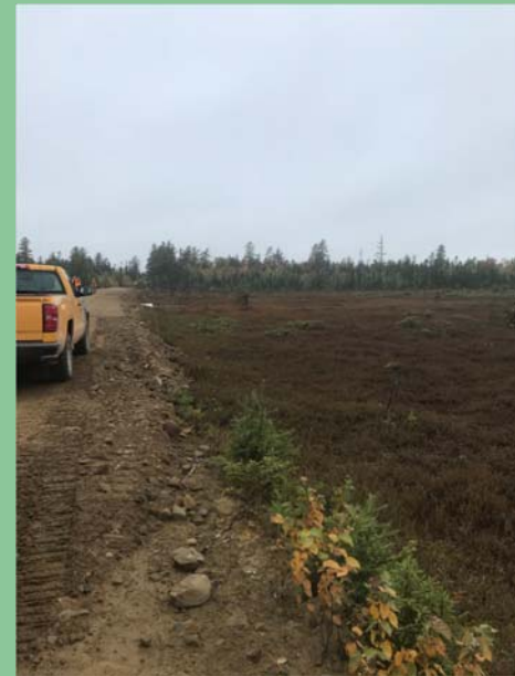
An example of an environmental upgrade undertaken on an old road crossing a wetland. The drainage has been improved to allow for improved water movement across the wetland.
